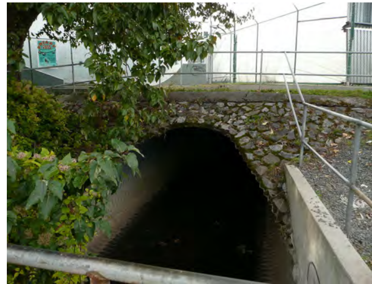
Culvert exiting from under the tennis bubbles at the top of Reach 3
