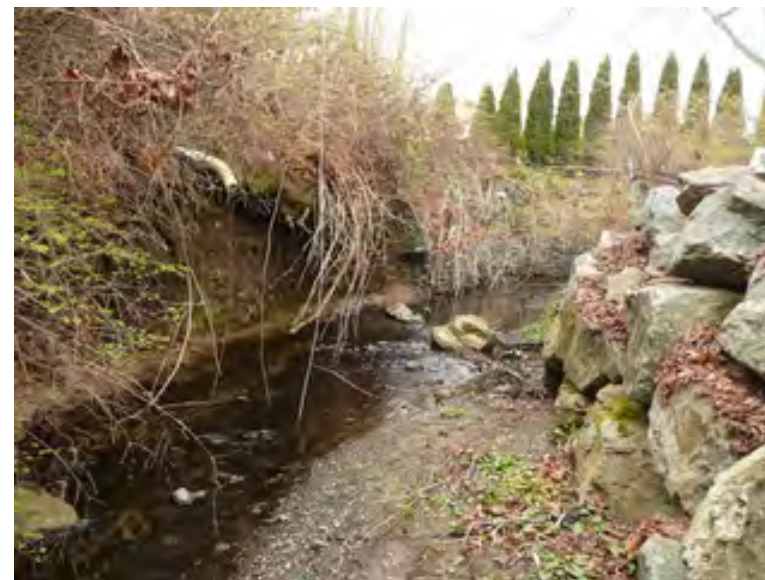
The section between McRae and North Dairy is constrained between private lots and has erosion issues.
