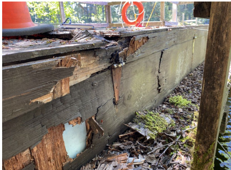
Figure 6: Insulated Casing and Deck Perimeter Severely Deteriorated.
