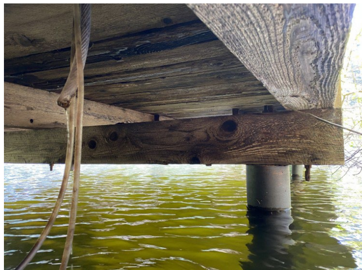
Figure 2: Underside of Deck Looking Towards the Lake – Steel Vertical Support Connecting to Wood Beam.
