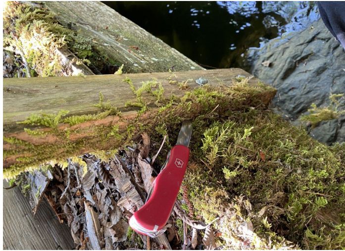
Figure 7: Wood Deck and Railing in Poor Condition.
