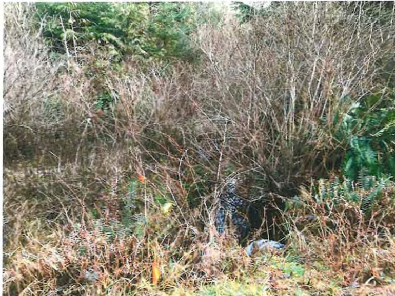
Photo 13: Invermuir Road roadside ditch connecting to Killecrankie Creek which crosses Invermuir Road via culvert.
