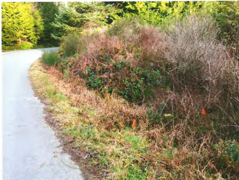
Photo 12. Ditch B is flows west along the northwest property line of 9333 Invermuir Road.
