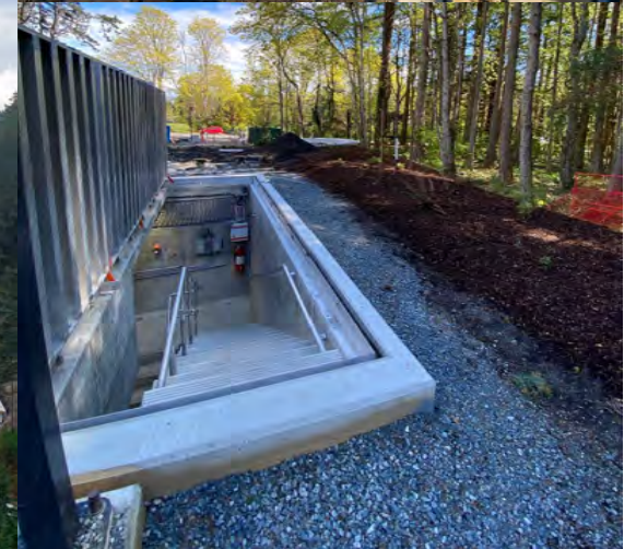
Arbutus Attenuation Tank
