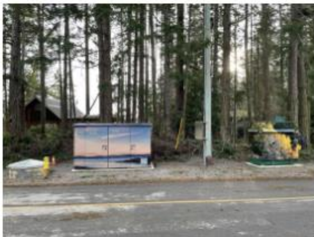
Schooner Pump Station and Genset
