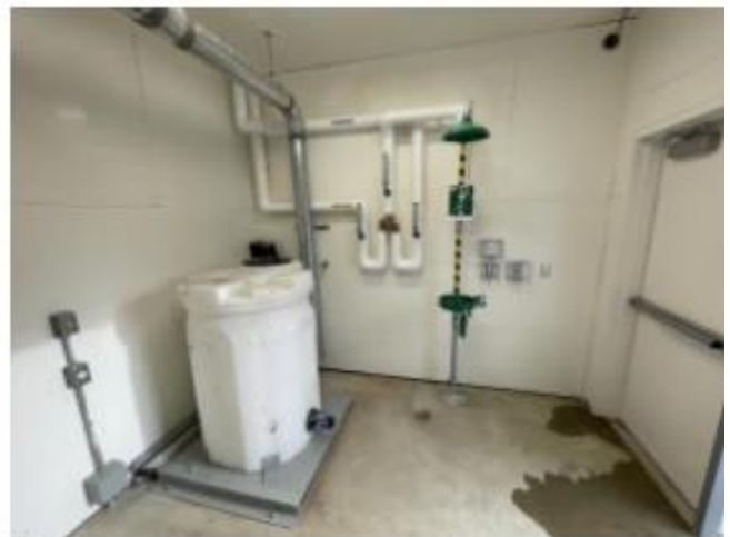
Chemical Clean Room
