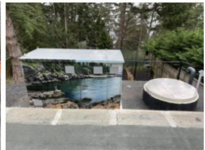
Cannon Pump Station
