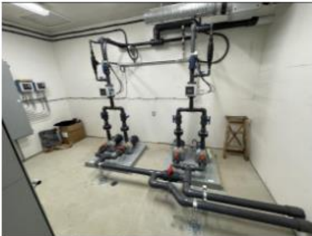
Permeate Pump Room
