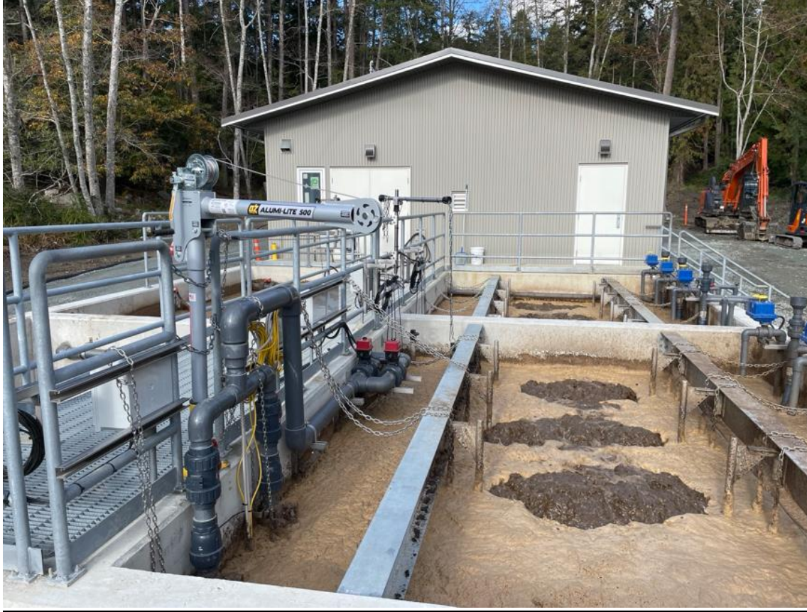
Schooner WWTP in Operation
