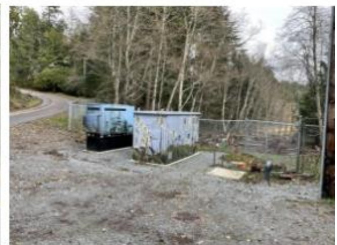
Galleon Pump Station and Genset
