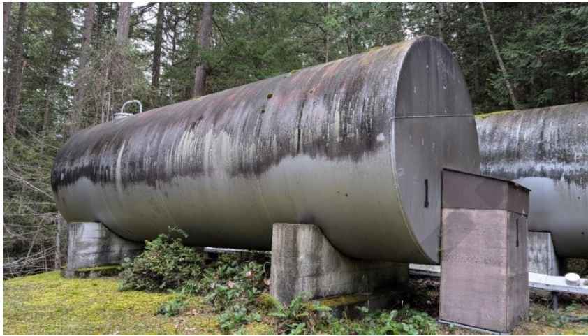
Figure 2-2 Skana Water Storage Tanks
