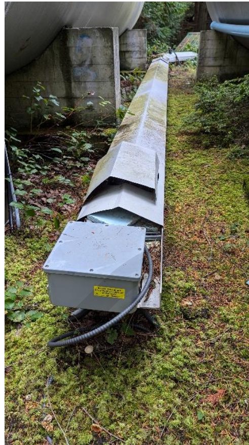
Figure B-3 Raceway Between Tanks
