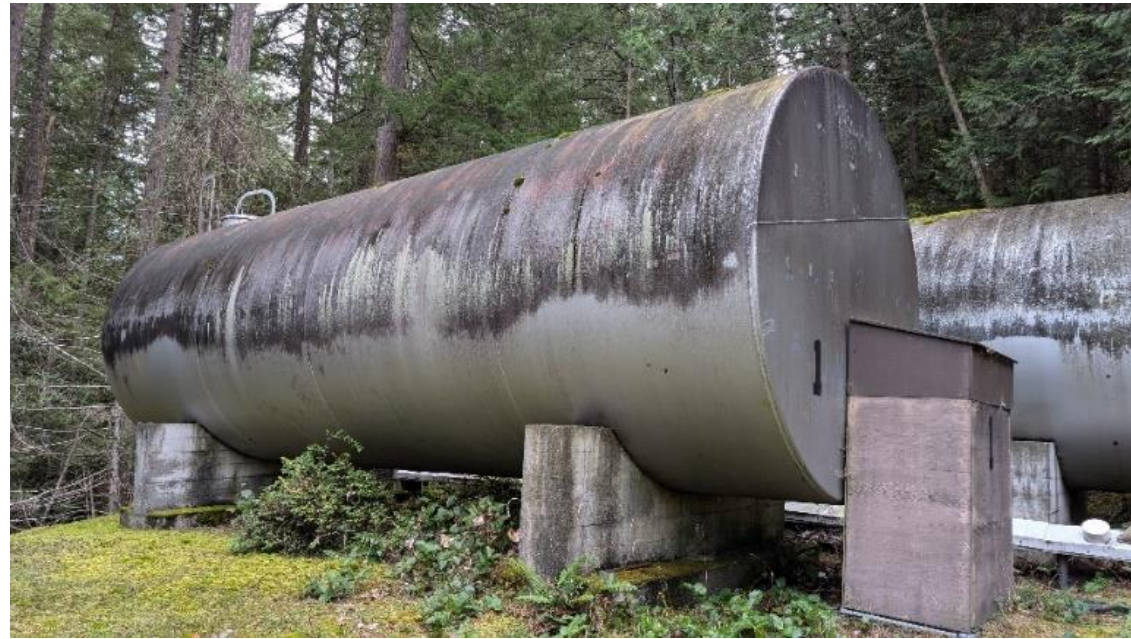
Figure B-1 Tank
