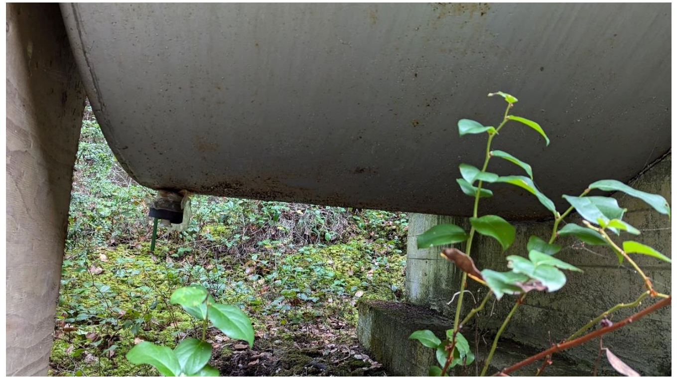
Figure B-8 Exterior Base of Tank 2
