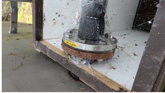
Figure B-4 Flange Connection/Corrosion
