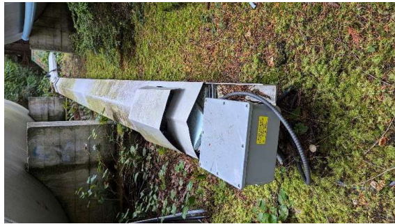
Figure B-3 Raceway Between Tanks
