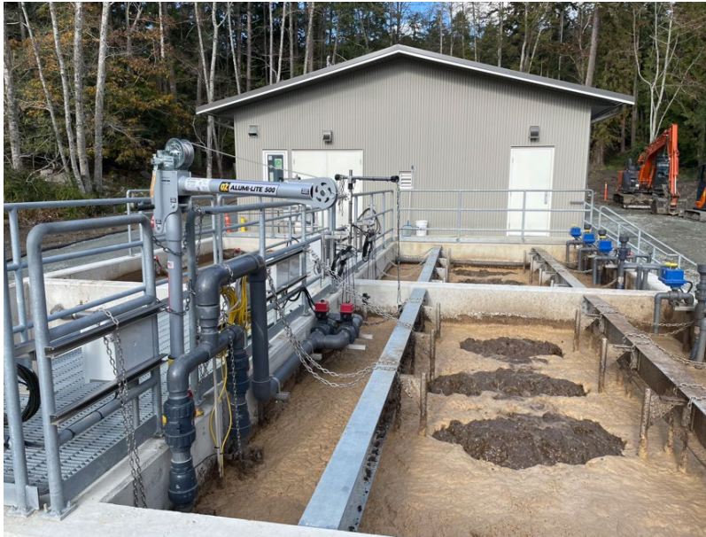
Schooner WWTP in Operation
