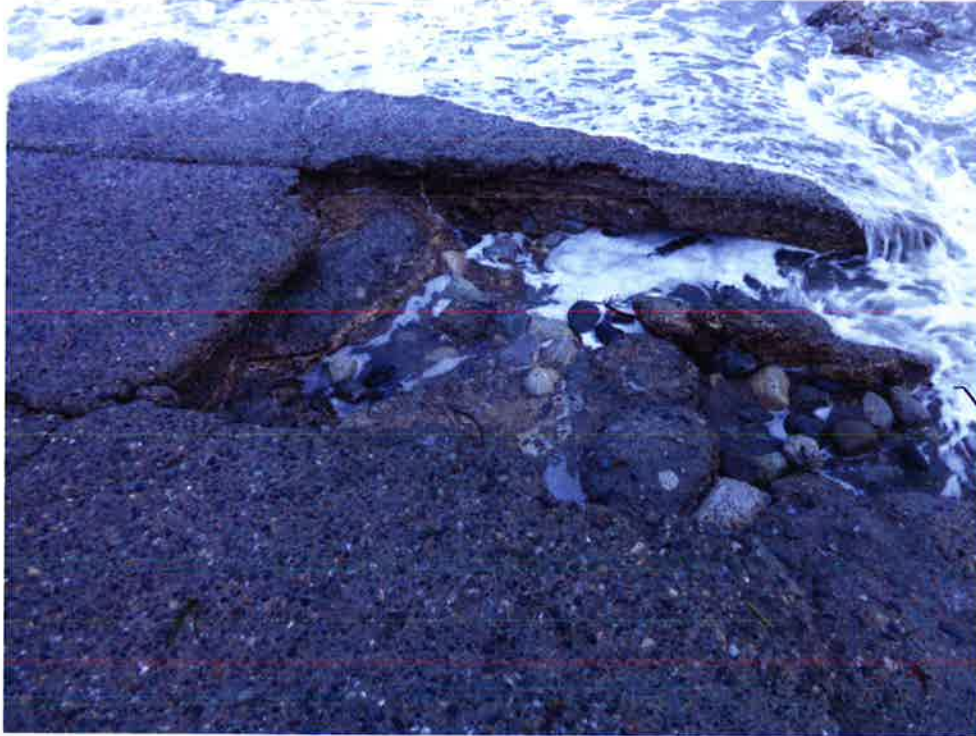
Photograph 8: Eroded surface of the boat ramp taken facing east on December 19, 2015
