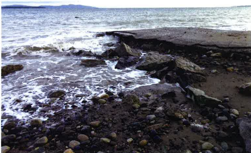
Photograph 7: The northern side of the boat ramp taken facing southeast on December 19, 2015
