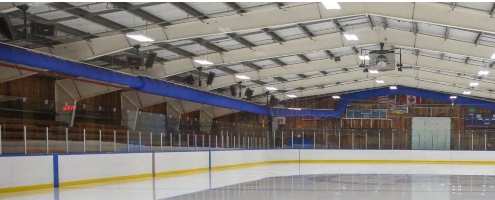
Panorama Recreation Arena B – Location of the ice plant and newly replaced dehumidifier, to be connected to the heat recovery system in 2026
