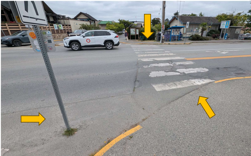
Figure 20: Lower Ganges / Hereford-Purvis Accessible Letdown Deficiencies
