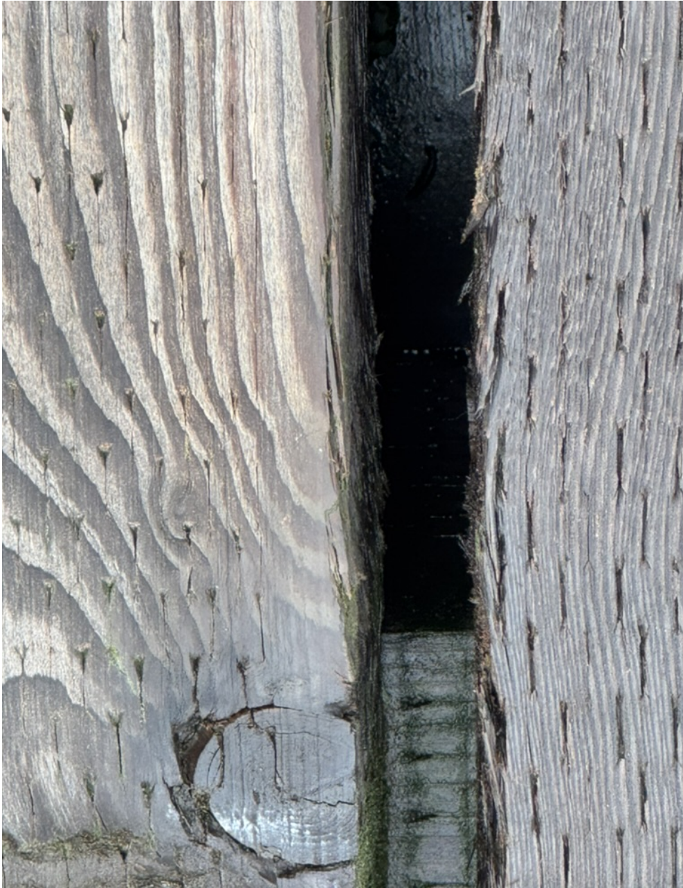
Drop strapping between dock planks
