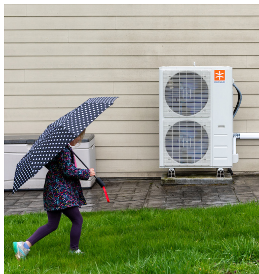
Heat pump outside family home
