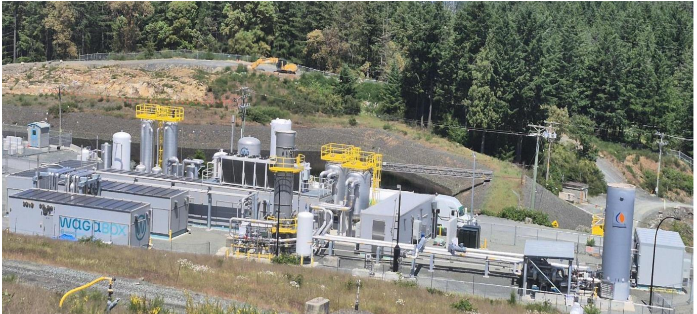
Biogas Upgrading Facility at Hartland Landfill
