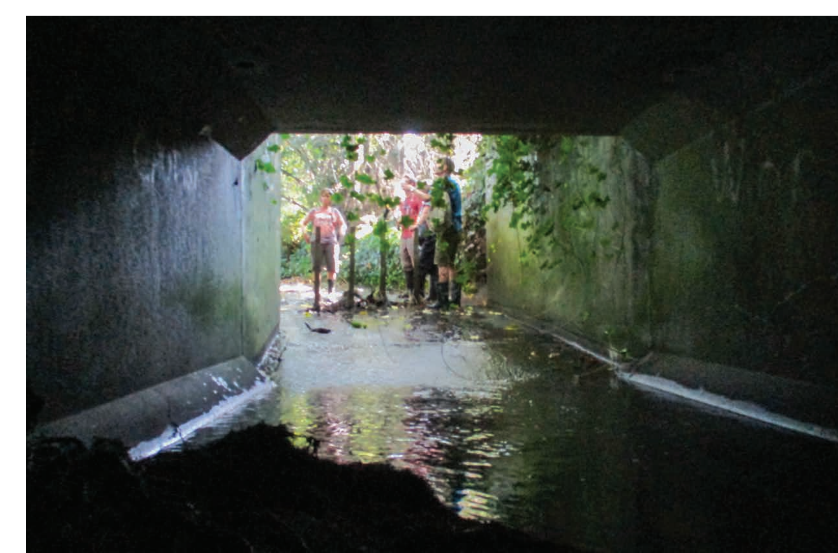
As the city grew across the watershed, Bowker Creek was put underground in pipes and stormwater from streets, roofs and parking lots directed into it.
