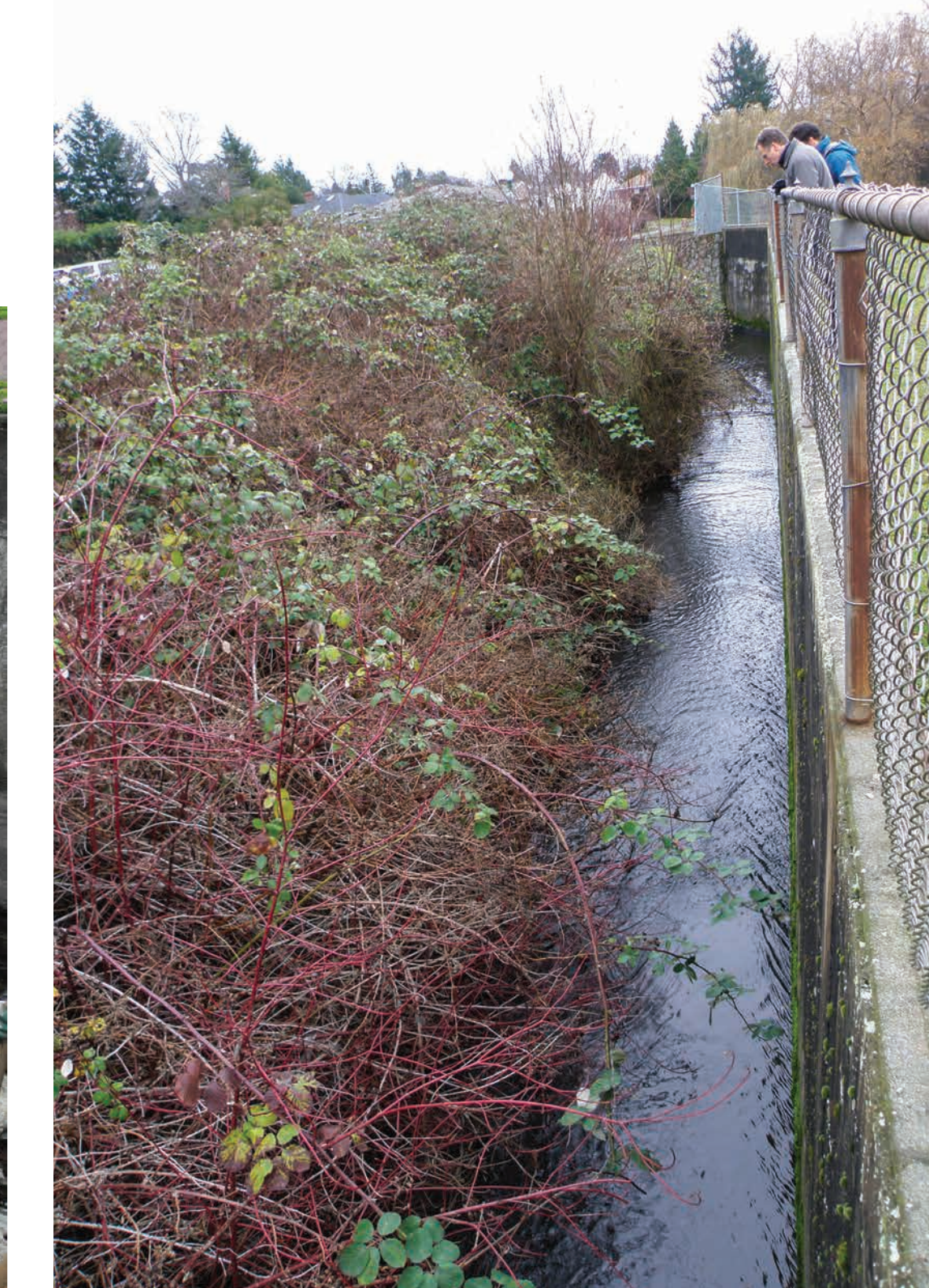
Before the restoration, Bowker Creek flowed through a narrow concrete channel, overgrown by invasive blackberries and golden willow.
