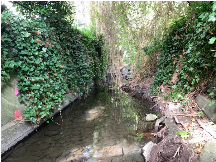
Upstream of the culvert at Beach Drive: English ivy on the concrete wall at 1762 Beach Drive, and eroding bank and english ivy at 1776 Beach Drive.
