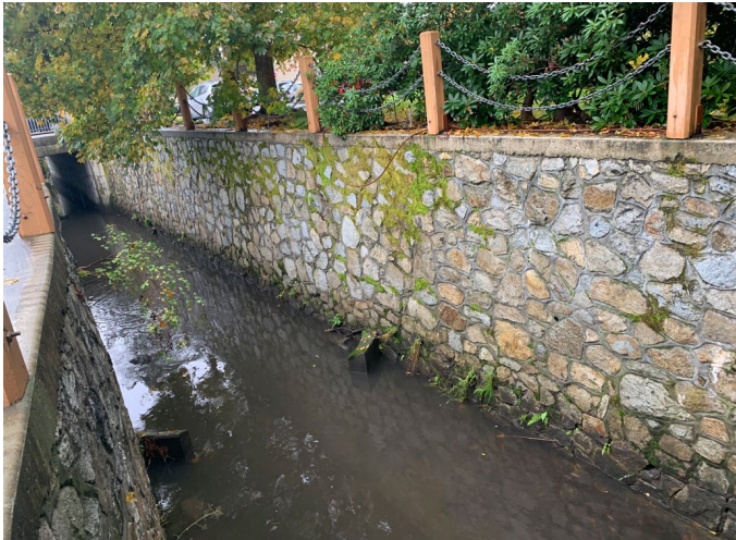
Vertical masonry walls and small incomplete weir with limited substrate complexity. Sword fern is growing from wall cracks.
