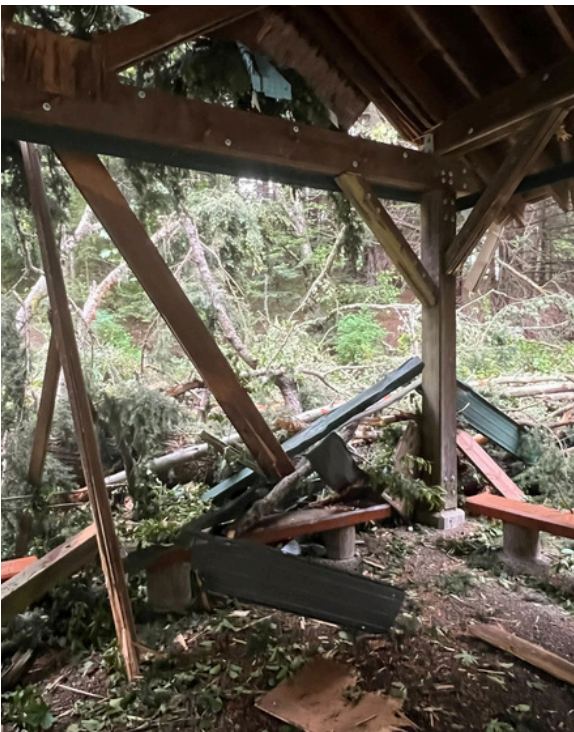
Damage to the Teaching Shelter from a fallen tree at Witty's Lagoon Regional Park at the end of May.
