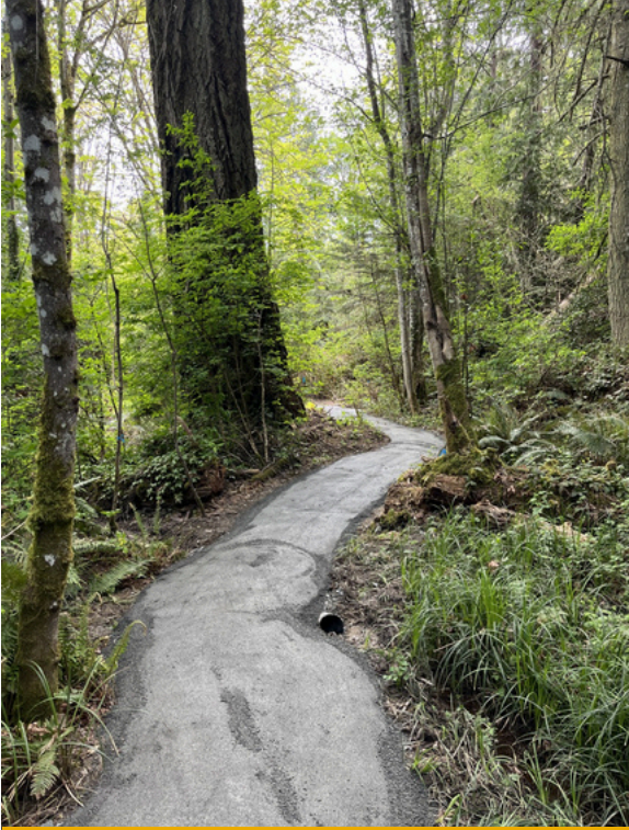
The newly constructed trail at Witty's Lagoon Regional Park after a landslide in the winter destroyed the original trail.
